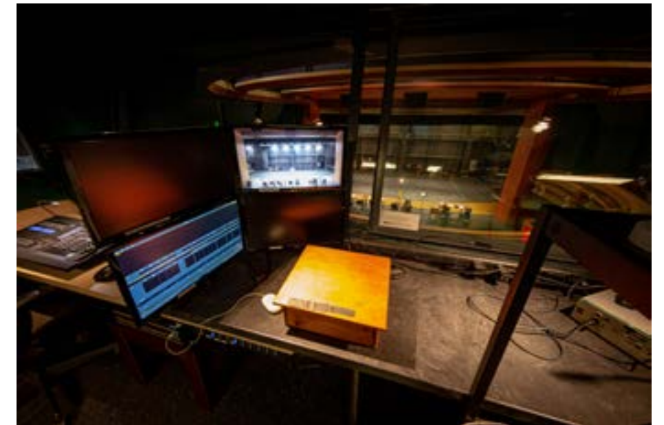
Stage Manager's station in control room
