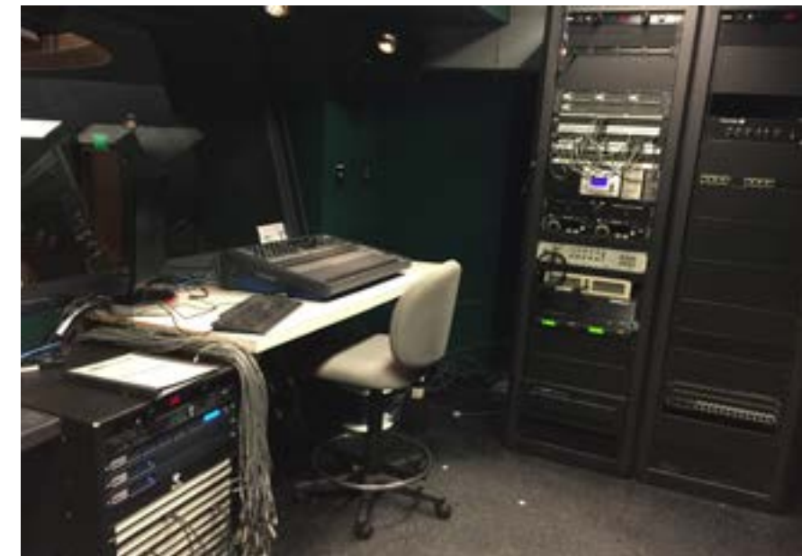
Audio Operator position in Control Room
